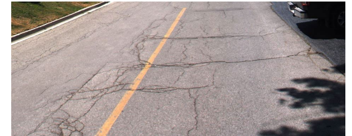
Poor Road Condition
